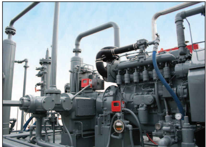
■ One of the initial packages with the VRC-2 driven by an Arrow VRG330 Cross Flow engine.
