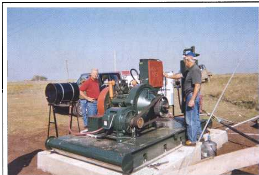
Since installing an induction generator system driven by a horizontal twin-cylinder engine capable of burning untreated high-Btu associated gas, Tidewater Petroleum has reduced lease electric costs by $2,000 a month in its Kay County, Ok., production operations. The wells average 20 barrels of oil a day or less and have high water cuts.
